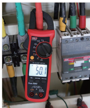
High voltage (600V) frequency measurement
